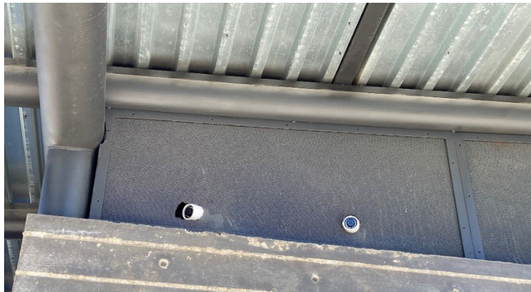
Figure 17: Digital camera installation at the CSRP pavilion for monitoring parking lot usage
