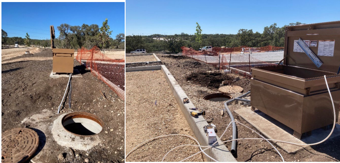
Figure 5: Manhole and instrumentation box
