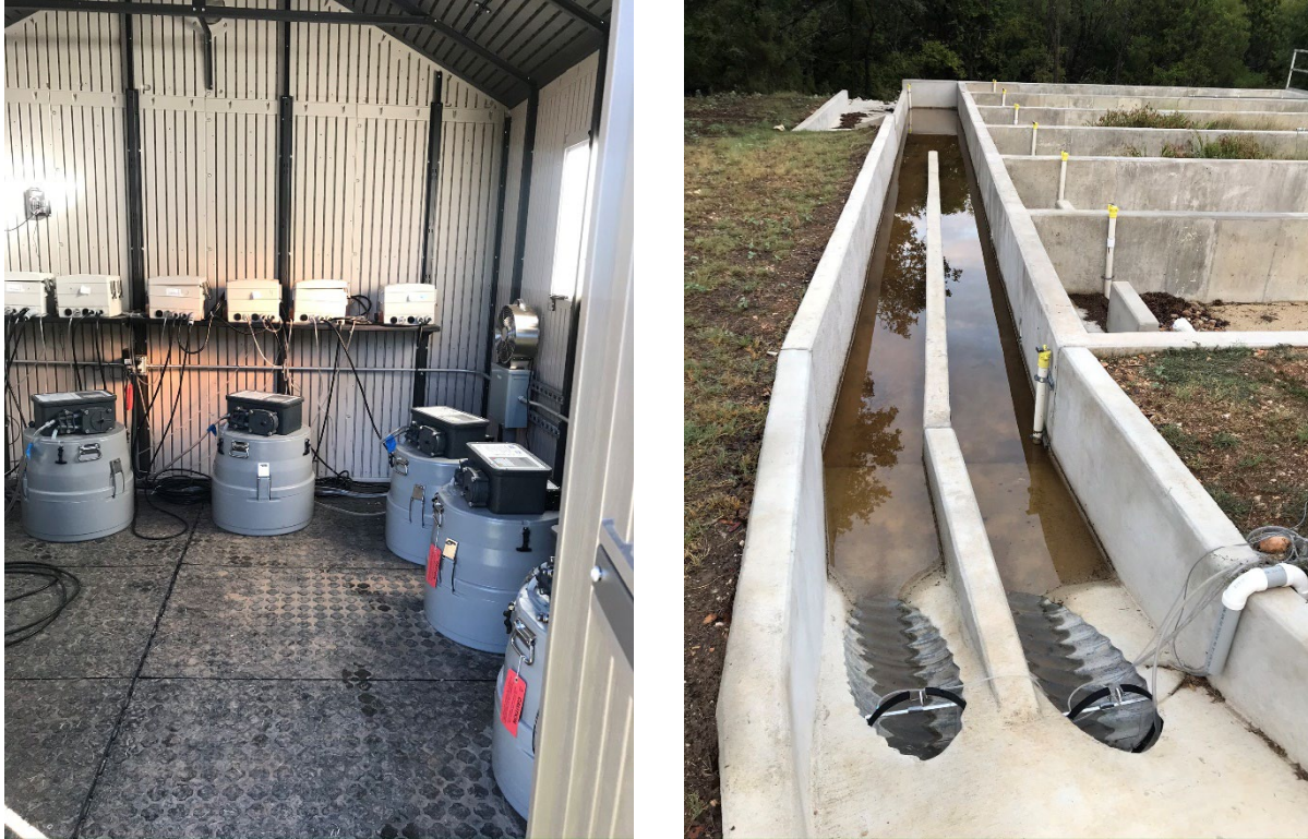
Figure 3- 4. Field monitoring equipment and sensors at the LID testbed
